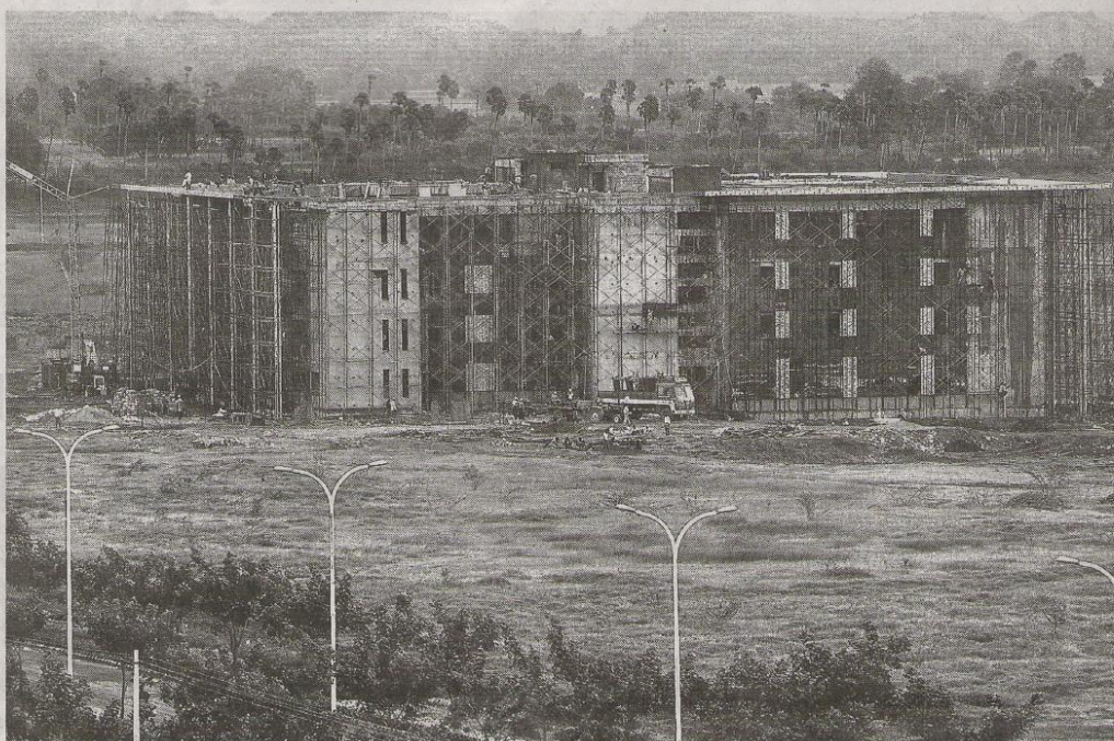
An upcoming software development centre of Infosys in Mahindra city at Maraimalai Nagar. — Photo: S.R. Raghunathan
